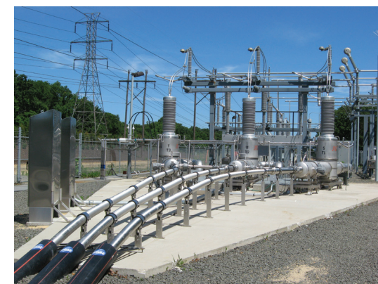
138 kV HTS cable system installed in Long Island, NY Image courtesy of American Superconductor
