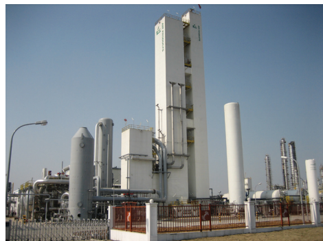
Large scale air separation unit in Nanjing Chemical Industrial Park (NCLIP), Eastern China Image courtesy of Air Products and Chemicals, Inc.
