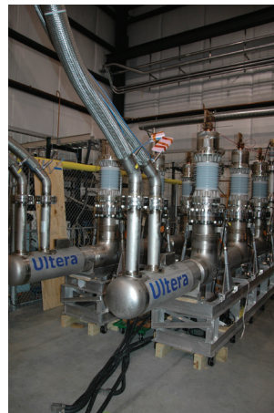
Type test of Project Hydra Fault Current Limiting 15 kV HTS TriaxTM Cable by Southwire, AMSC, ORNL, Con Edison, DHS Image courtesy of Southwire
